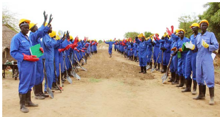
LIPW beneficiaries at the Ritnhom access road in Bor County. This road connects farmers to market opportunities in Bor County and beyond. Photo: Janet Maya Logo / Ministry of Agriculture and Food Security.
